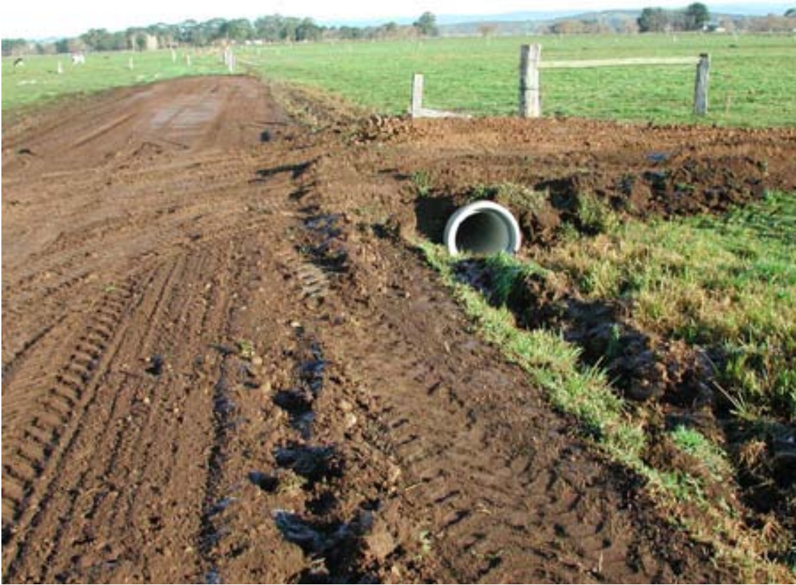
A farm track under construction. Adequate allowance has been made for drainage and the base material is being crowned and compacted using a vibrating roller
